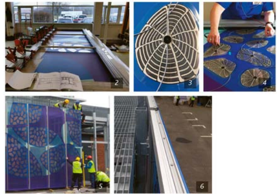
Figure 2: Assembly of the 64 frames in Taiyo Europe's workshop (standard size 4.2x1.3m, as shown here; special size 4.2x0.5m) Figure 3: OPV-modules glued on the backside.
