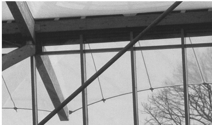
Fig. 2: Public bath PRIENAUVERA, Prien at Lake Chiemsee, canopy, 1999, ETFE-film single layer structure, mechanically pre-stressed, cable-supported, NOWOFOLON ET6235 200 \mu\text{m} , 17 fields, total surface area: approx. 200 \text{m}^2 , field-size approx. 12 \text{m}^2 in average, architect: ZELLER & ROMSTÄTTER, Traunstein, Structural Design and Engineering: ZELLER, Traunstein, TENSYS Ltd. Bath/UK, realization membrane roof: Koch Membrane Structures GmbH, Rimsting [3]
